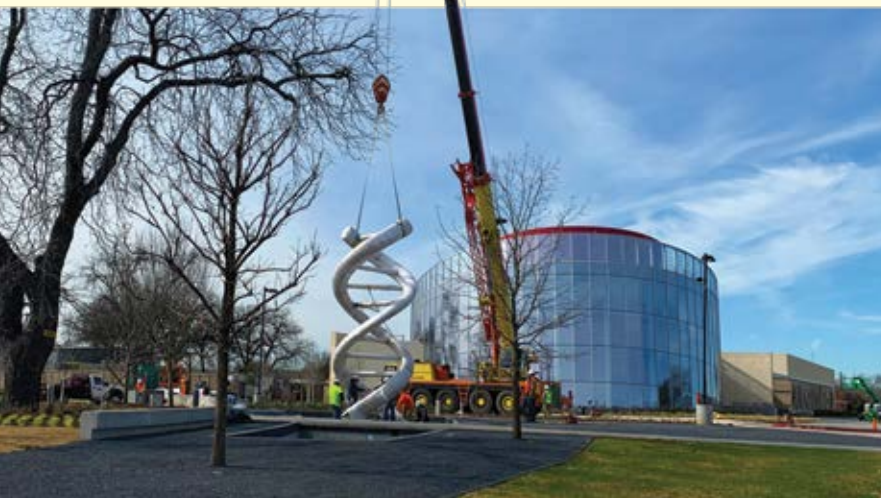
A crane sets in place the 24-foot steel DNA sculpture that marks the entrance to the Discovery Center and outdoor park
